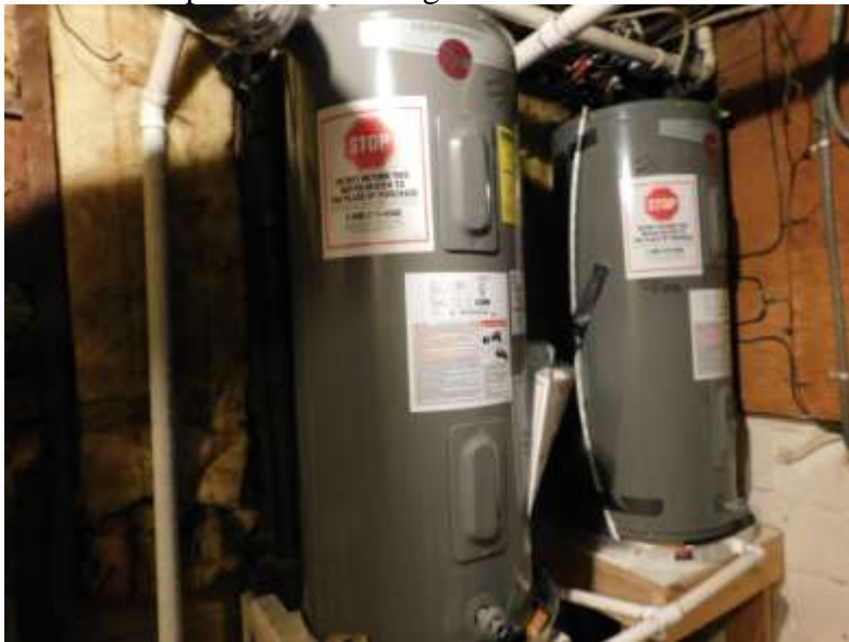
First Floor Apartment Building – Water Heaters 1 & 2
