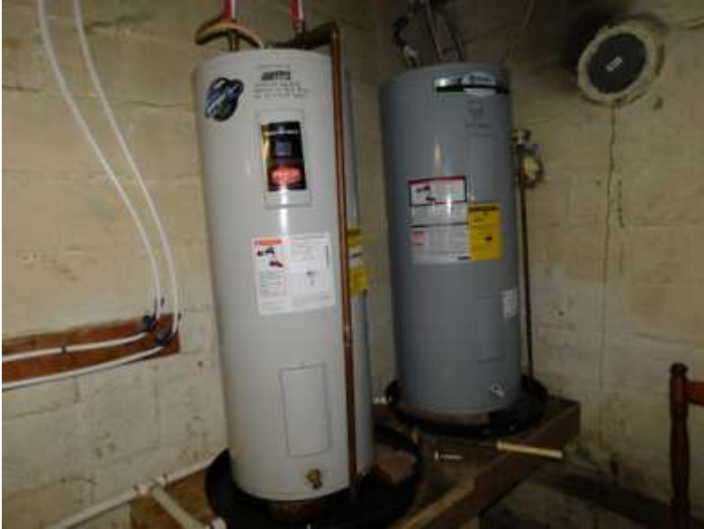
First Floor Apartment Building – Water Heaters 3 & 4
