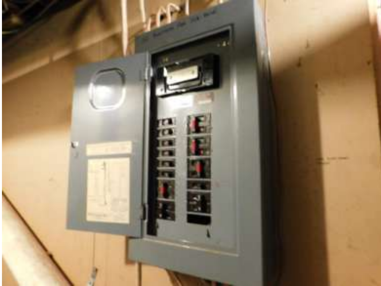
First Floor Apartment Building – Additional Electrical Panel Box
