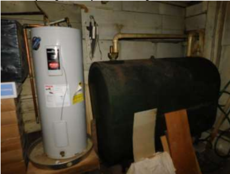
Accessory Single Family Unit Building Unit R1 – Water Heater & Oil Tank
