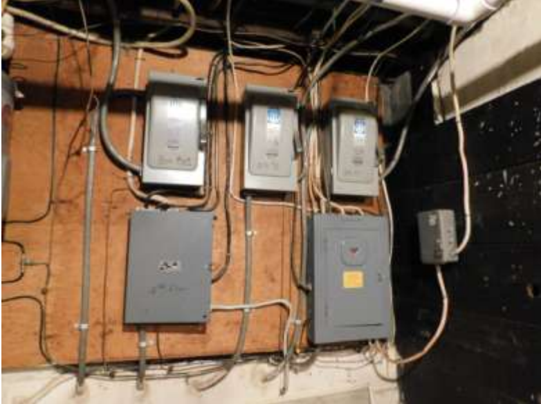
First Floor Apartment Building – Electrical Panel Boxes
