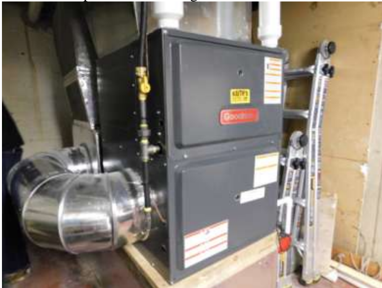
First Floor Apartment Building – Propane Gas Fired Furnace
