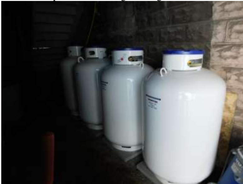
Propane Tanks for Apartment Building
