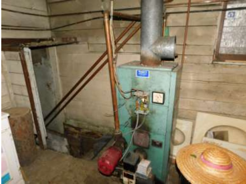
Accessory Single Family Unit Building Unit R1 – Furnace
