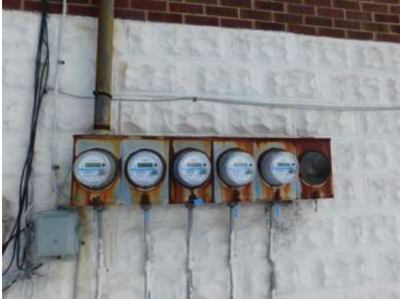
Separate Electric Meters for Apartment Building
