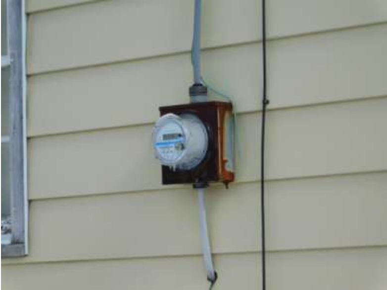
Electric Meter for Single Family Unit Accessory Building
