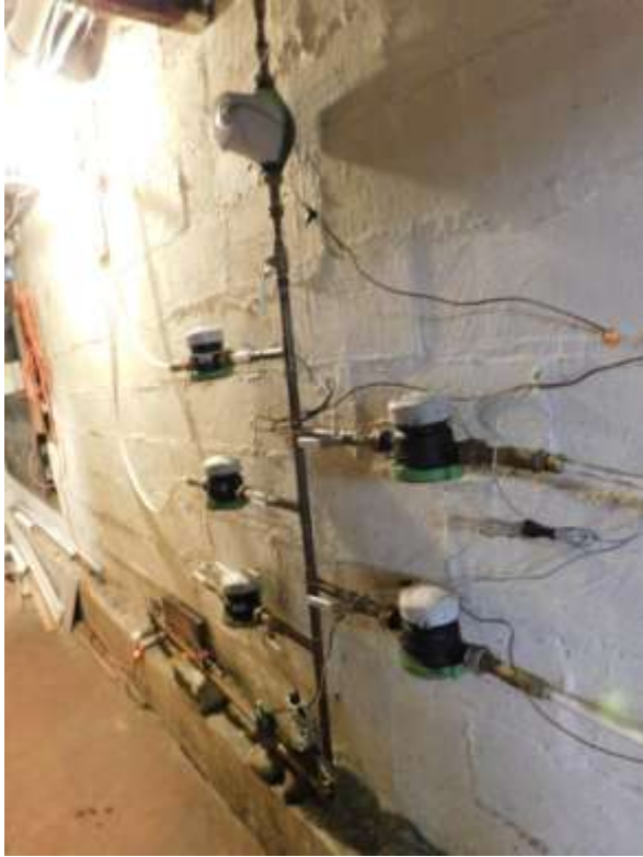
First Floor Apartment Building – Water Meters
